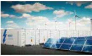
Energy Storage System
